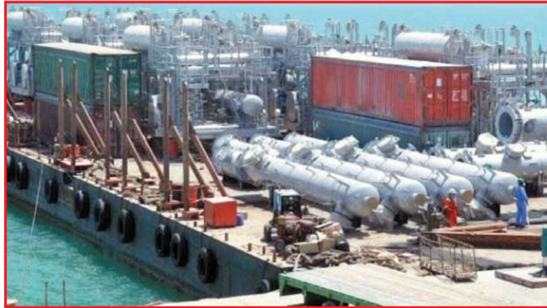
● Work under way on installing seven new gas dehydration units at Bapco
